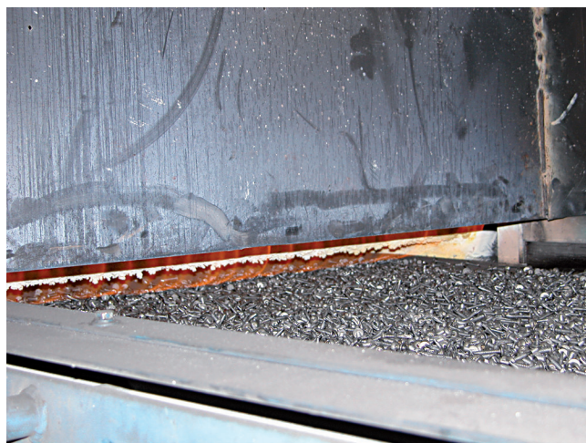
Fig. 1 — Wet/oily parts entering a heat treat furnace.
